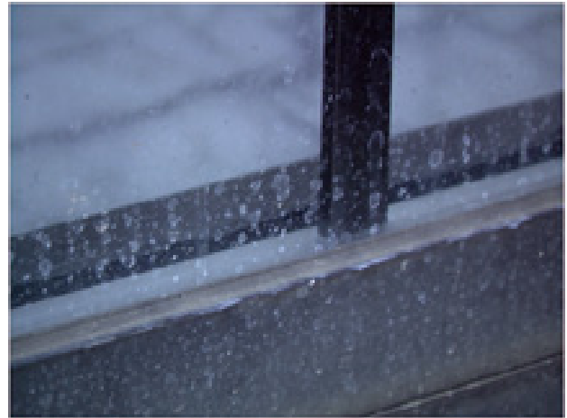
Figure 15 Hard water spots containing silicate materials after normal attempts at cleaning.
