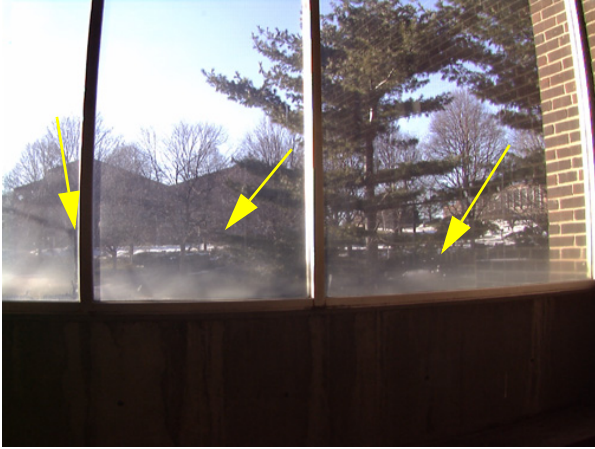
Figure 9: Visible gray haze due to deposits on glass from concrete runoff. Implementation of conventional cleaning procedures failed to remove deposits.
