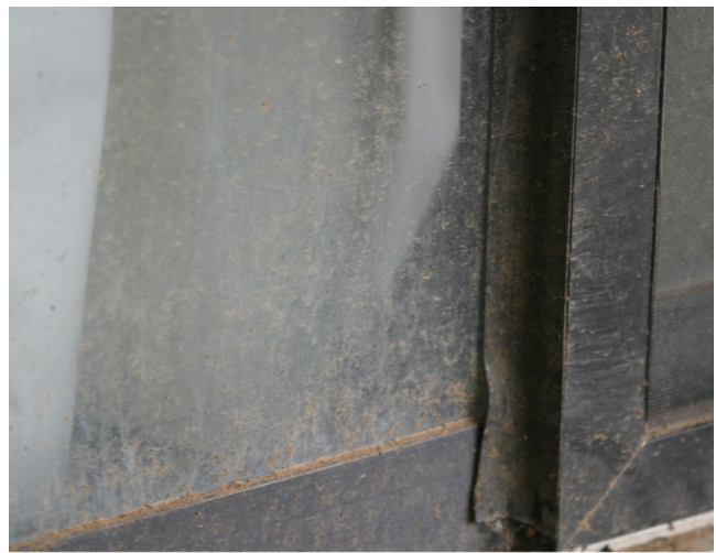
Fig. 5: Close-up view of dirt and soil on window at
