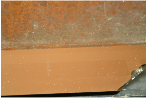
Figure 12. Concrete runoff deposits on coated glass unit removed from an existing glazing installation. Note the line of demarcation at point where glass was protected by framing.
